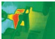
Motor: cojinete defectuoso
